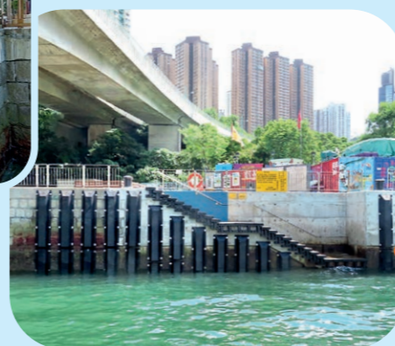
在鴨脷洲北增設公眾登岸梯級 Additional public landing steps at ALC North
